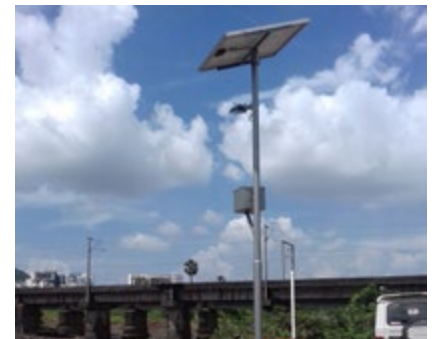
Installed Solar Street Light in Panvel
