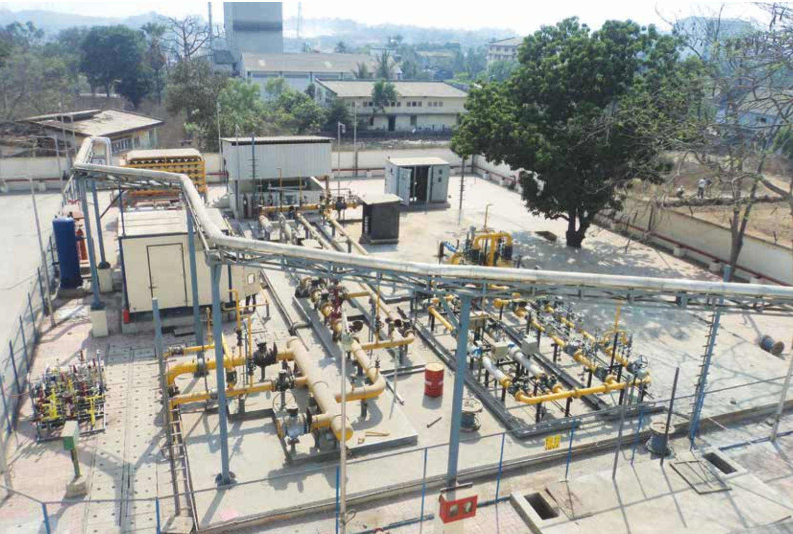
City Gate Station, Mahape.
