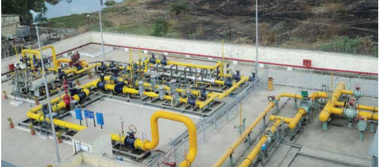
City Gate Station, Ambarnath.
