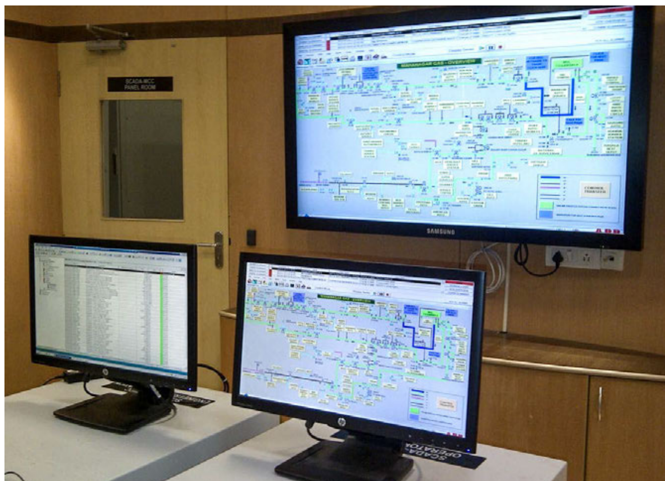
SCADA system at MGL
