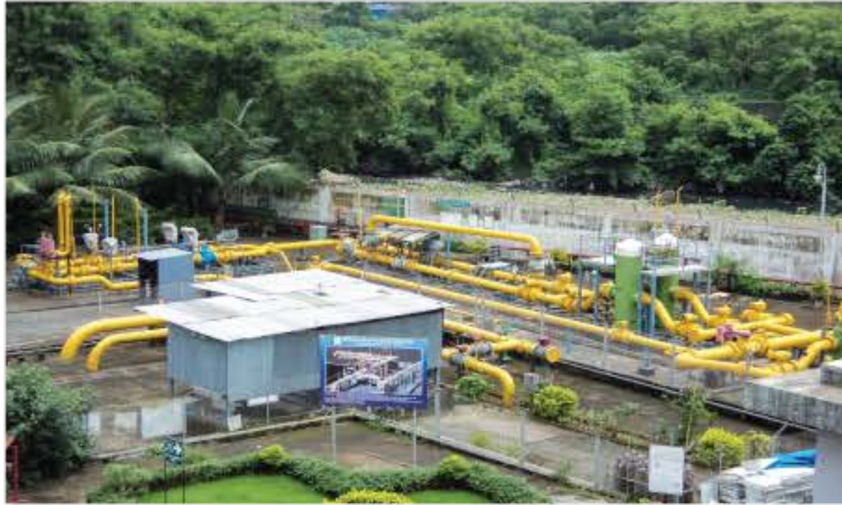
City Gate Station, Wadala
