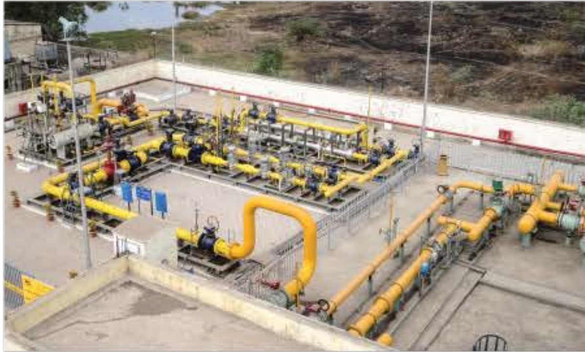
City Gate Station, Mahape
